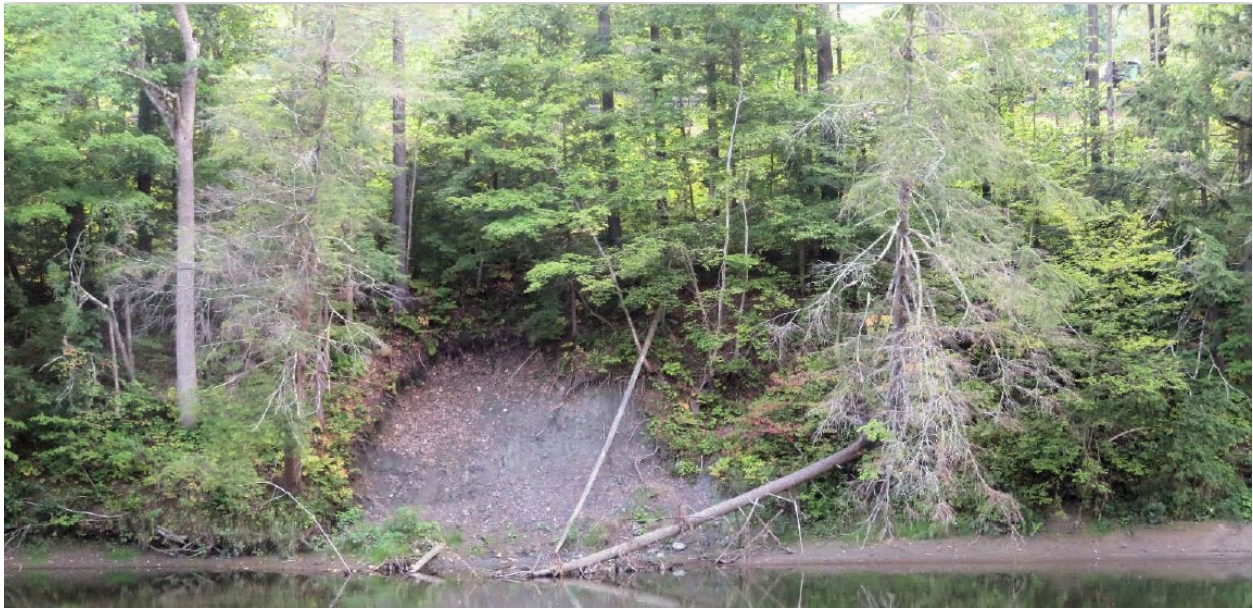
Photo 3-7 Slumped Soils on Right Bank below U.S. Route 4 in August 2024, first observed in 2023 (GMP 2024)
