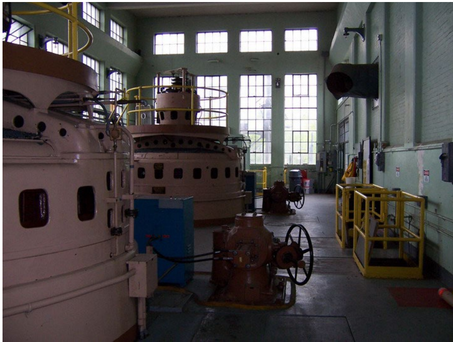
Photo 2.3 View of powerhouse interior and generating units.
