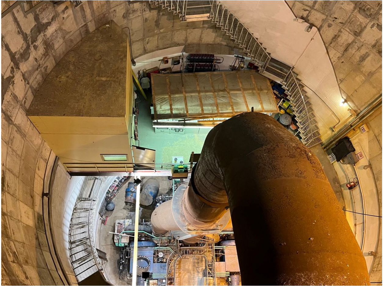
Figure 6. Mt Ida Project Facilities (Powerhouse) (Interior)
