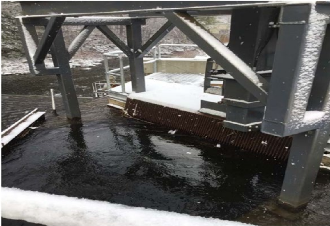
Figure 10. Trash Racks at Intake of Newbury Project.
