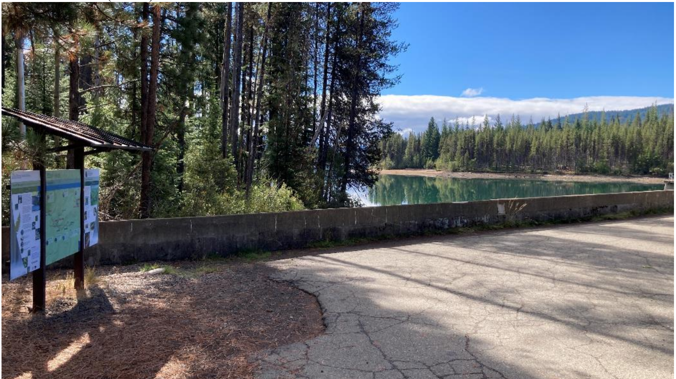
Photo 2. Looking southeast from the right abutment of Lemolo No. 1 Dam at the downstream extent of Lemolo Reservoir (ZOE 1). FPA Part 8 recreation signage is seen at left of frame.
