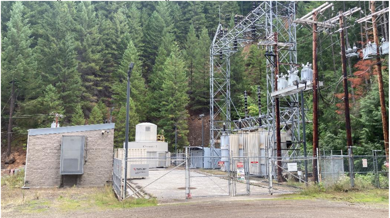
Photo 22. Looking east at Clearwater No. 2 powerplant, which discharges flows to Toketee Reservoir (ZOE 5) from the southeastern shoreline.
