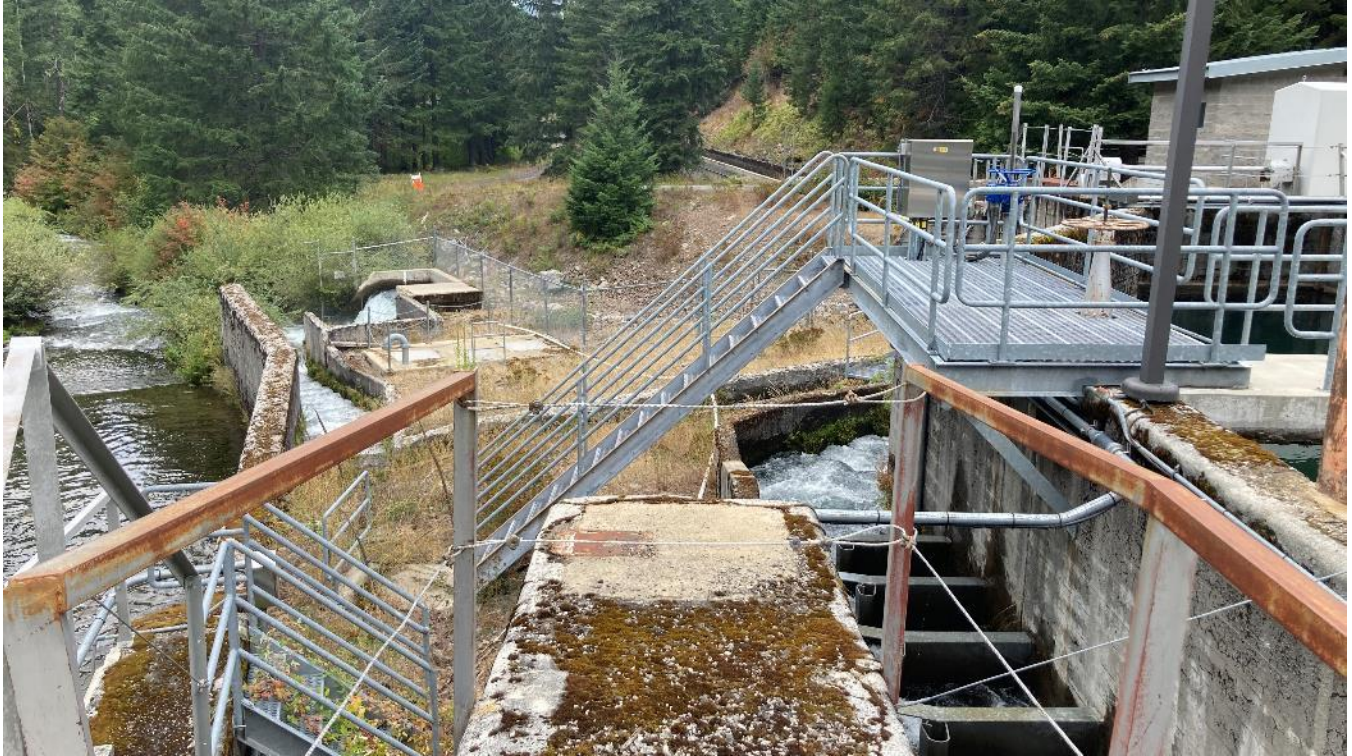
Photo 13. Looking downstream (west) from Lemolo No. 2 dam at the Lemolo No. 2 fish ladder. The upper Lemolo No. 2 bypassed reach (ZOE 4) is seen at the left of frame.
