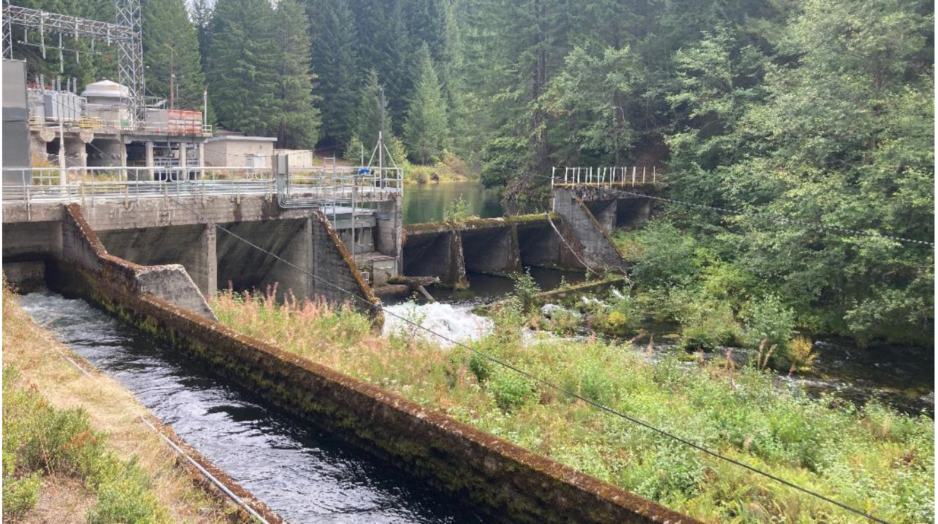
Photo 39. Looking upstream (east) at the transition from the lower Clearwater No. 1 bypassed reach (ZOE 14; middle distance) to the Clearwater No. 2 impoundment (ZOE 15) upstream of Clearwater No. 2 dam. Clearwater No. 2 powerplant is seen at left of frame. Clearwater No. 2 bypassed reach (ZOE 16) is seen at the middle right of frame.
