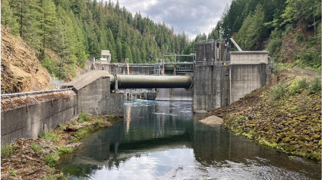
Photo 33. Looking upstream (southeast) at Soda Springs Dam and the upper Soda Springs bypassed reach of the North Umpqua River (ZOE 11). The fish ladder entrance can be seen at water level on the center left of frame. The fish screen structure is at the right of frame. Freshly installed spawning gravels are seen at the base of the fish screen.
