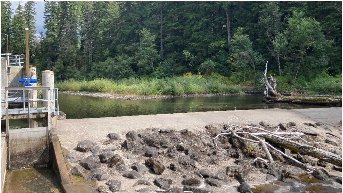
Photo 42. Looking east (upstream) at Fish Creek impoundment (ZOE 17) and Fish Creek dam. The fish ladder exit and diversion intake are seen at left of frame.
