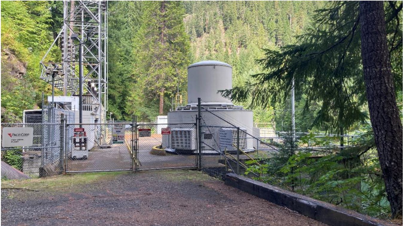
Photo 27. Looking north at Fish Creek powerplant. Slide Creek impoundment (ZOE 7) can be seen through the trees at lower right of frame. The Slide Creek dam spillway gate can be seen to the right of the generator.
