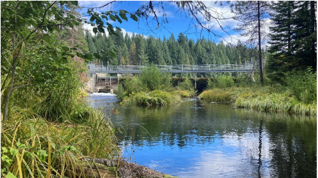
Photo 38. Looking northeast (upstream) at Clearwater No. 1 dam and the upper Clearwater No. 1 bypassed reach of Clearwater River (ZOE 14).
