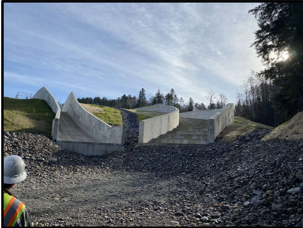
Figure 11: Molly's Falls Reservoir Emergency Spillway (right), Service Spillway (left), and plunge pool (foreground)
