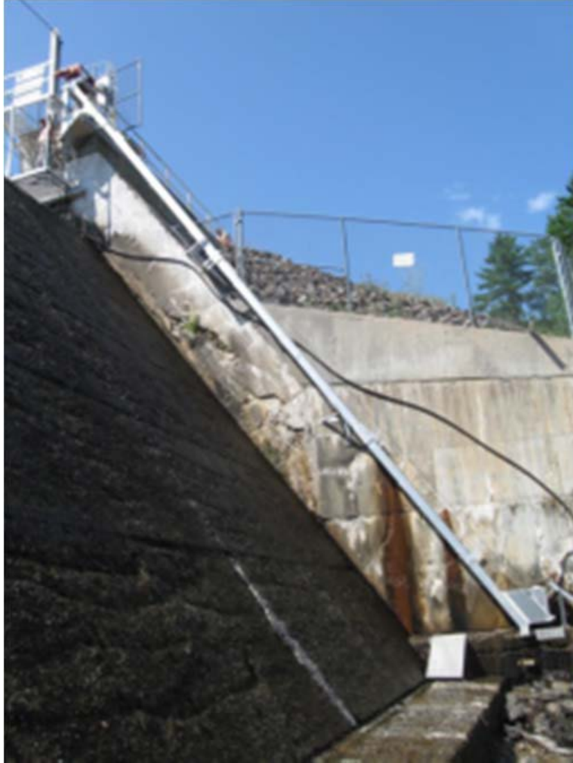
Upstream Eel Passage Lift
