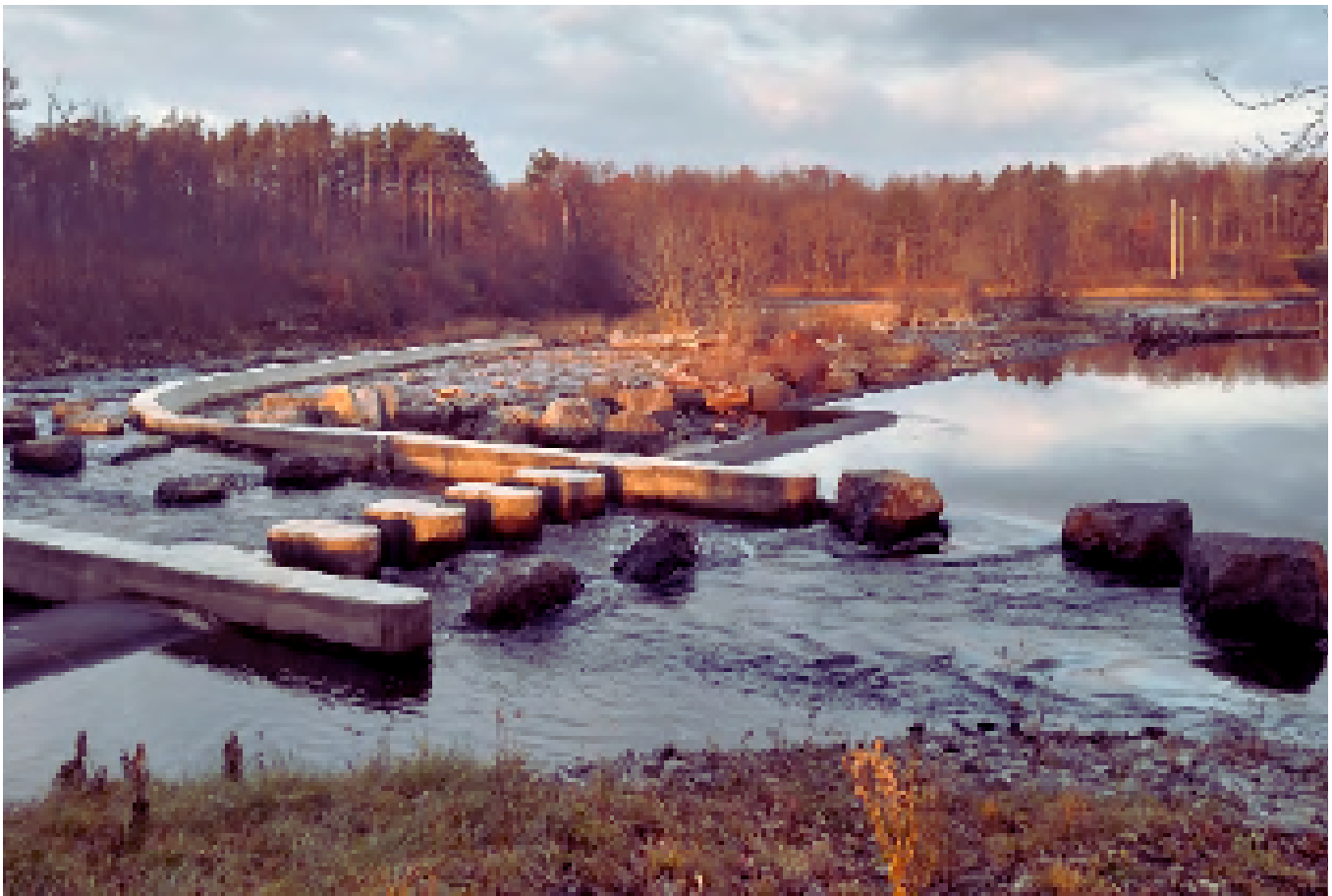
Figure 7. Boulders and cement blocks mimic natural riverbed conditions, allowing multiple fish species to pass upstream and downstream of the Eel Weir project safely 5 .
