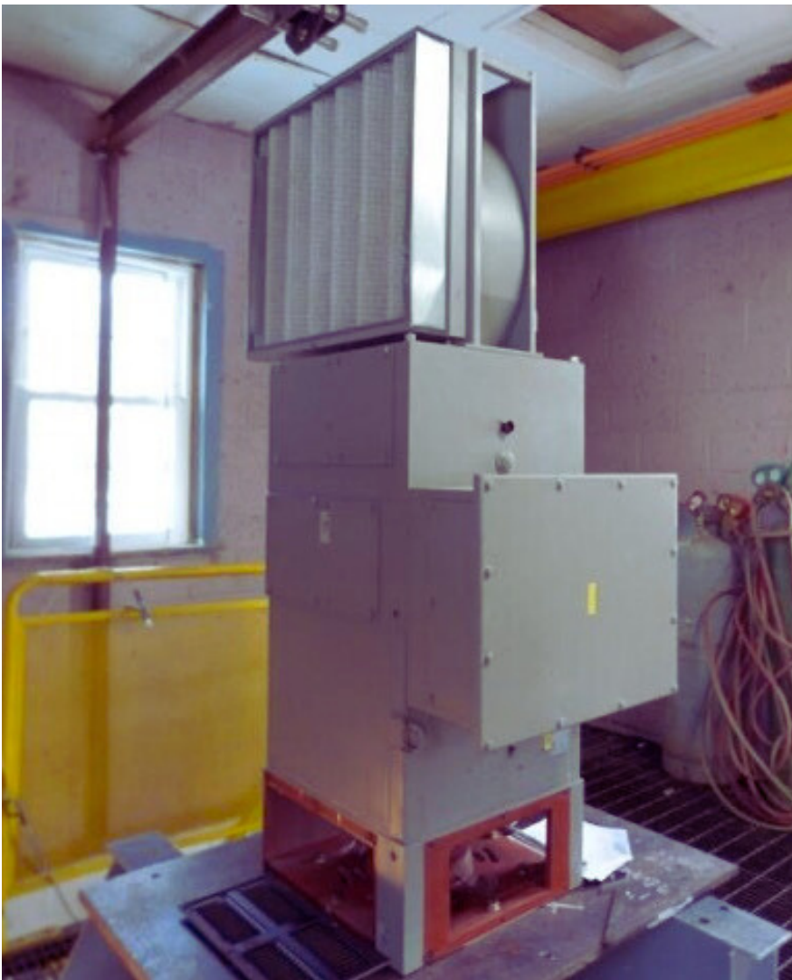
Figure 6. While nondescript, the magnet generator shown here (gray) connects to the turbine shaft below.
