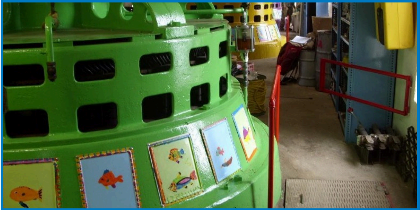
Figure 10. Artwork created by the local 4th-grade class adds beauty to the powerhouse and creates a learning environment for future school kids.
