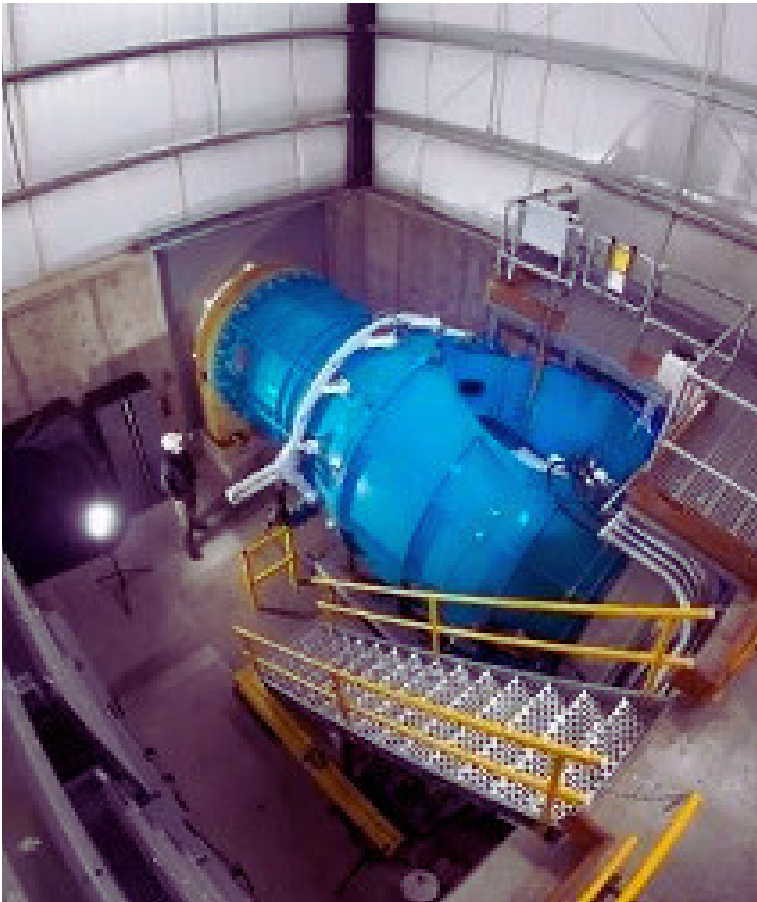
Figure 5. Natel Restoration Turbine (blue) sits between the intake to the right and discharge to the left of the Monroe Drop Project.
