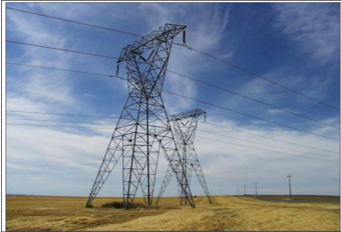
Figure 4. 230-kV transmission lines of the Wells Project
