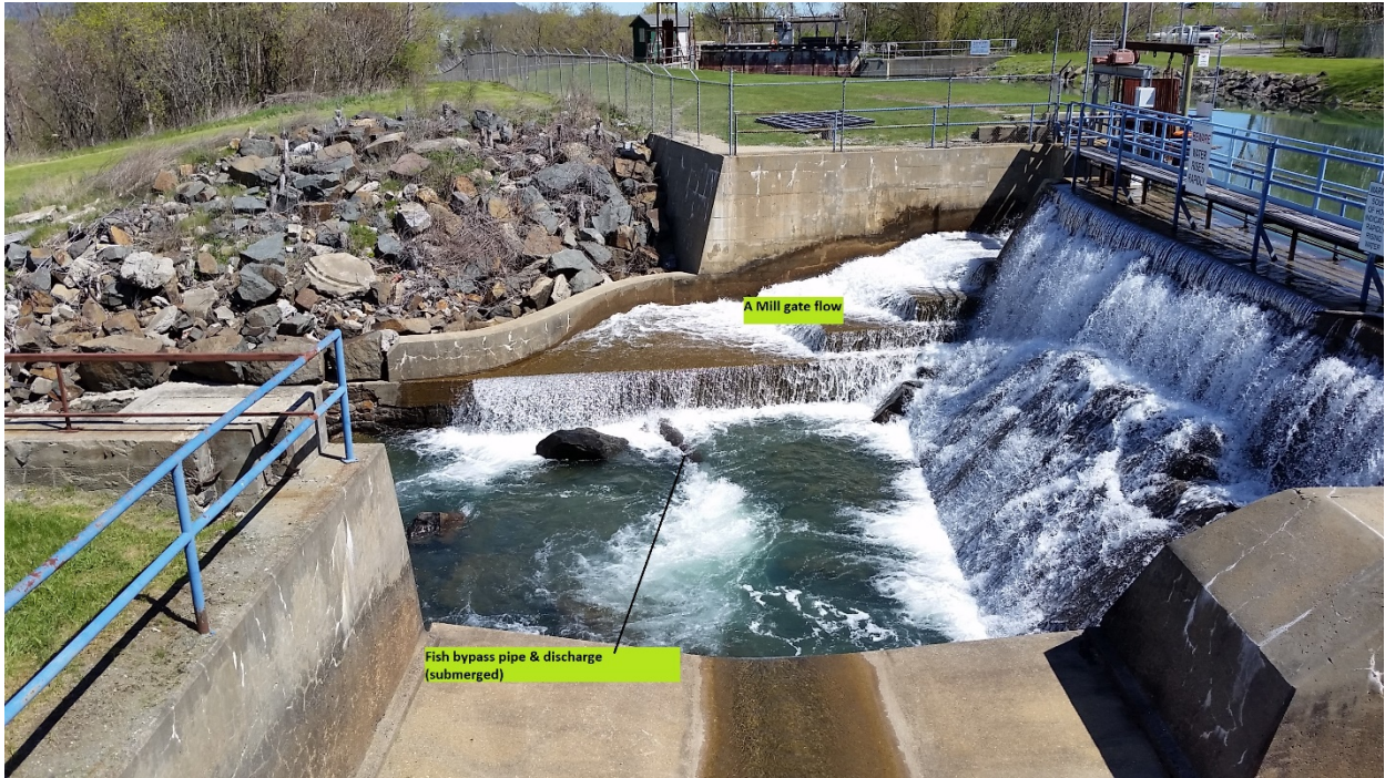
Upper project, A-Mill dam min flow: gate flow plus fish bypass discharge. See also LIHI Stage 1 Application photo 1.1.
