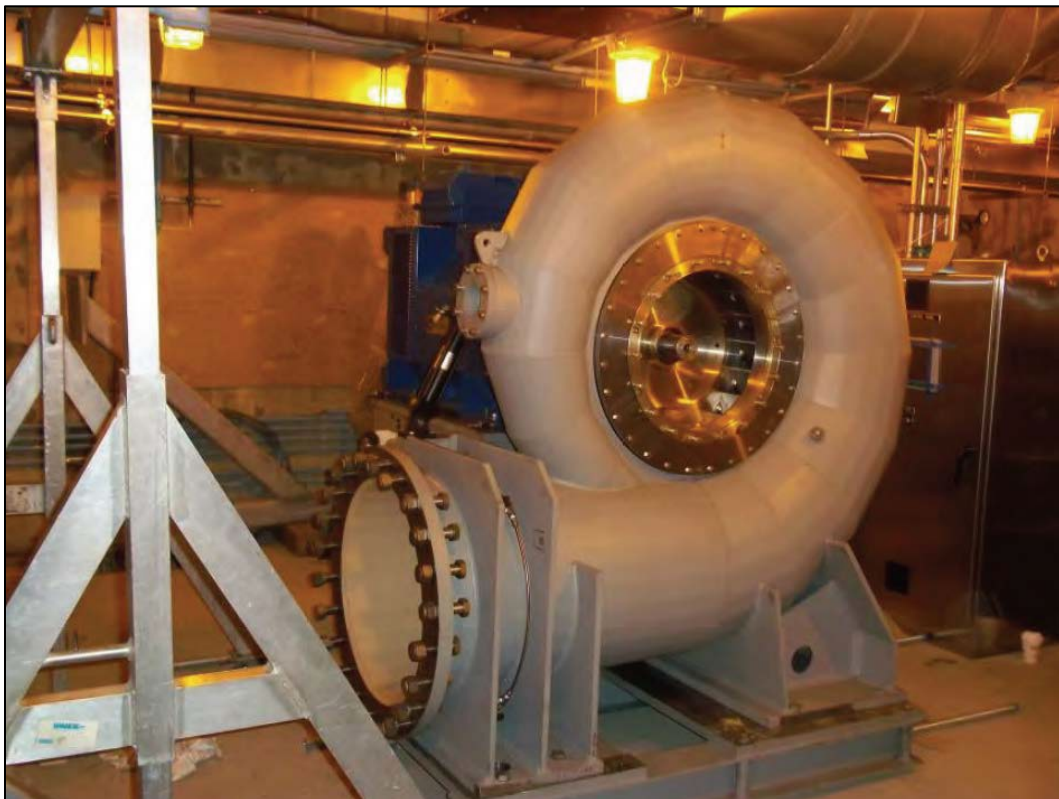
Photo 1: Horizontal Francis Turbine at Loring Road Facility
