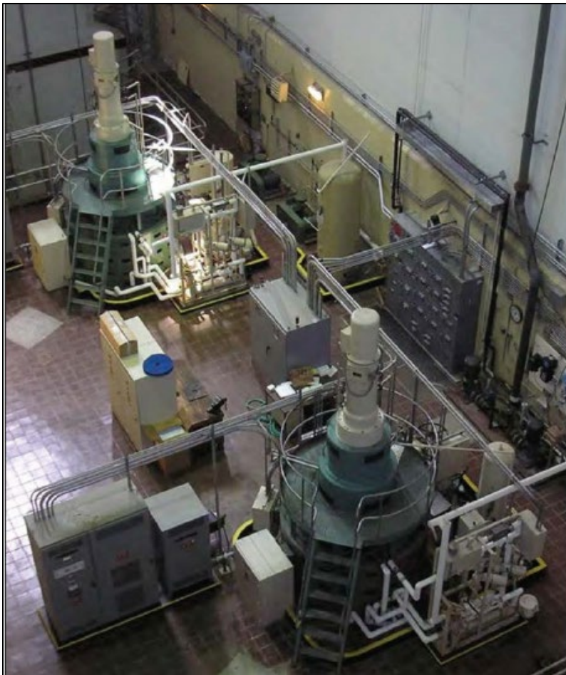
Photo 1: Kaplan Turbine at Cosgrove Project
