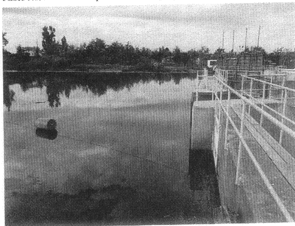
Photo No. 10 - View of upstream warning sign on concrete wall adjacent to the barrier at Dam No. 18.
