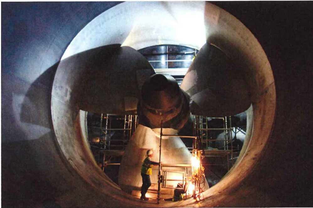
Figure 4. Horizontal Axis Bulb Turbine (note the person standing inside).
