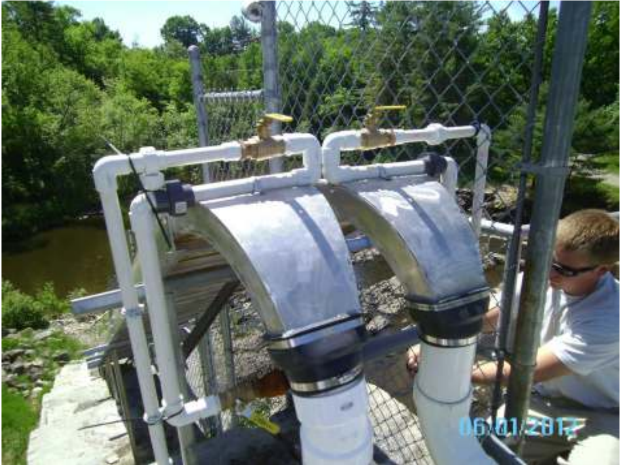
Terminal ends with plumbing and exit pipes.
