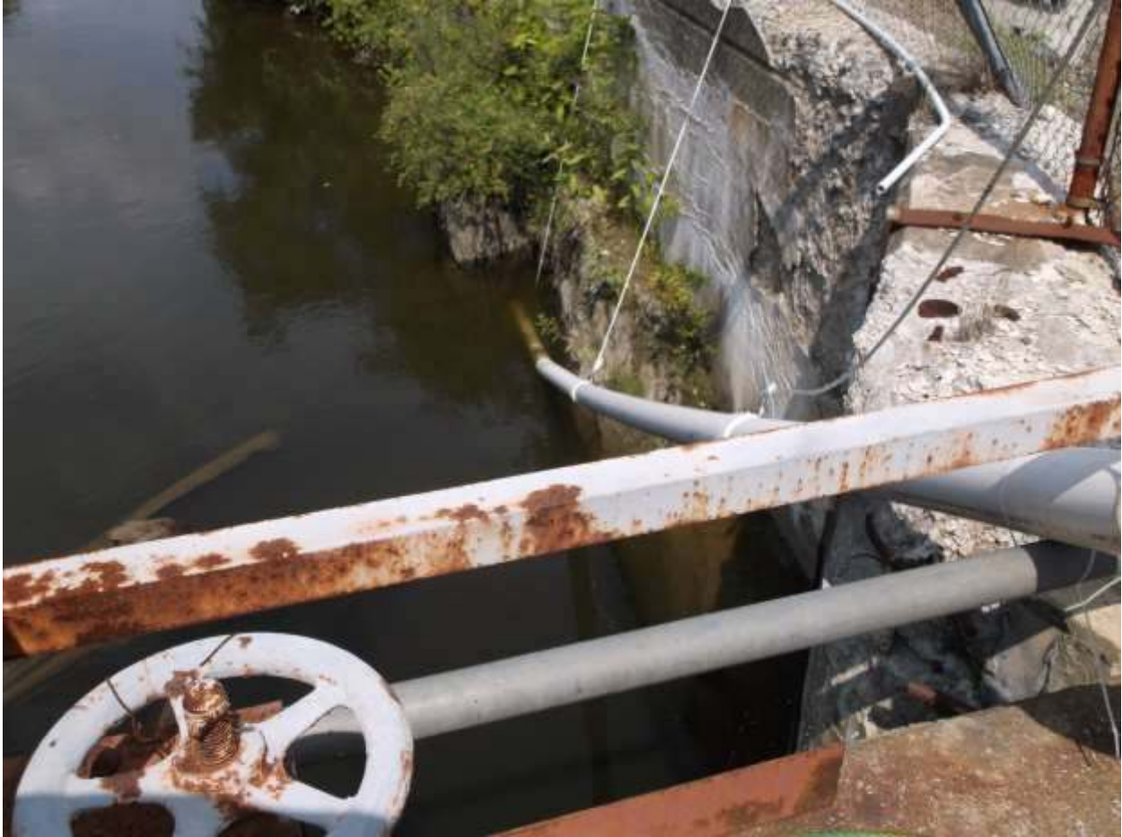
Head pond exit pipe location
