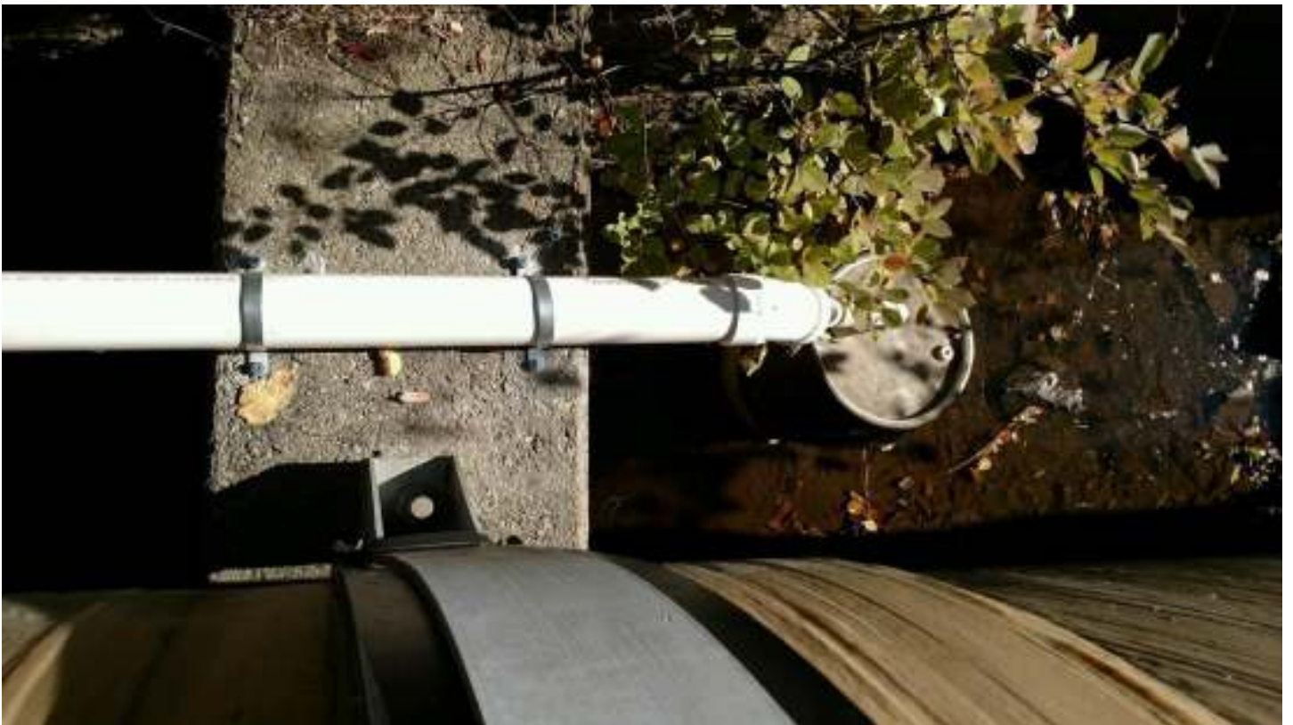
Exit pipe into catch tank
