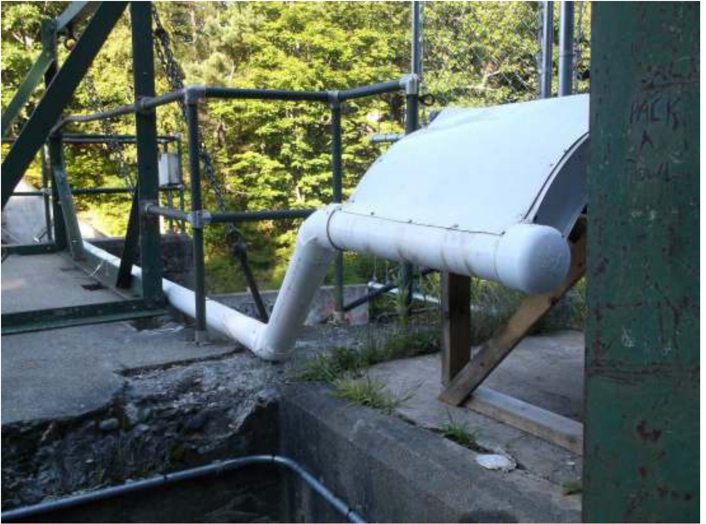
Piping across minimum flow gate
