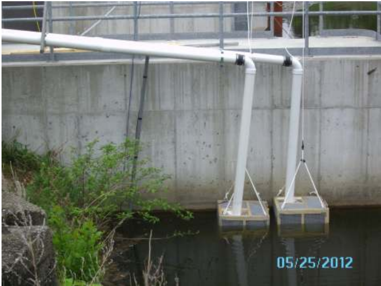
Holding pens, with exit pipes in place, and plumbing from pump.
