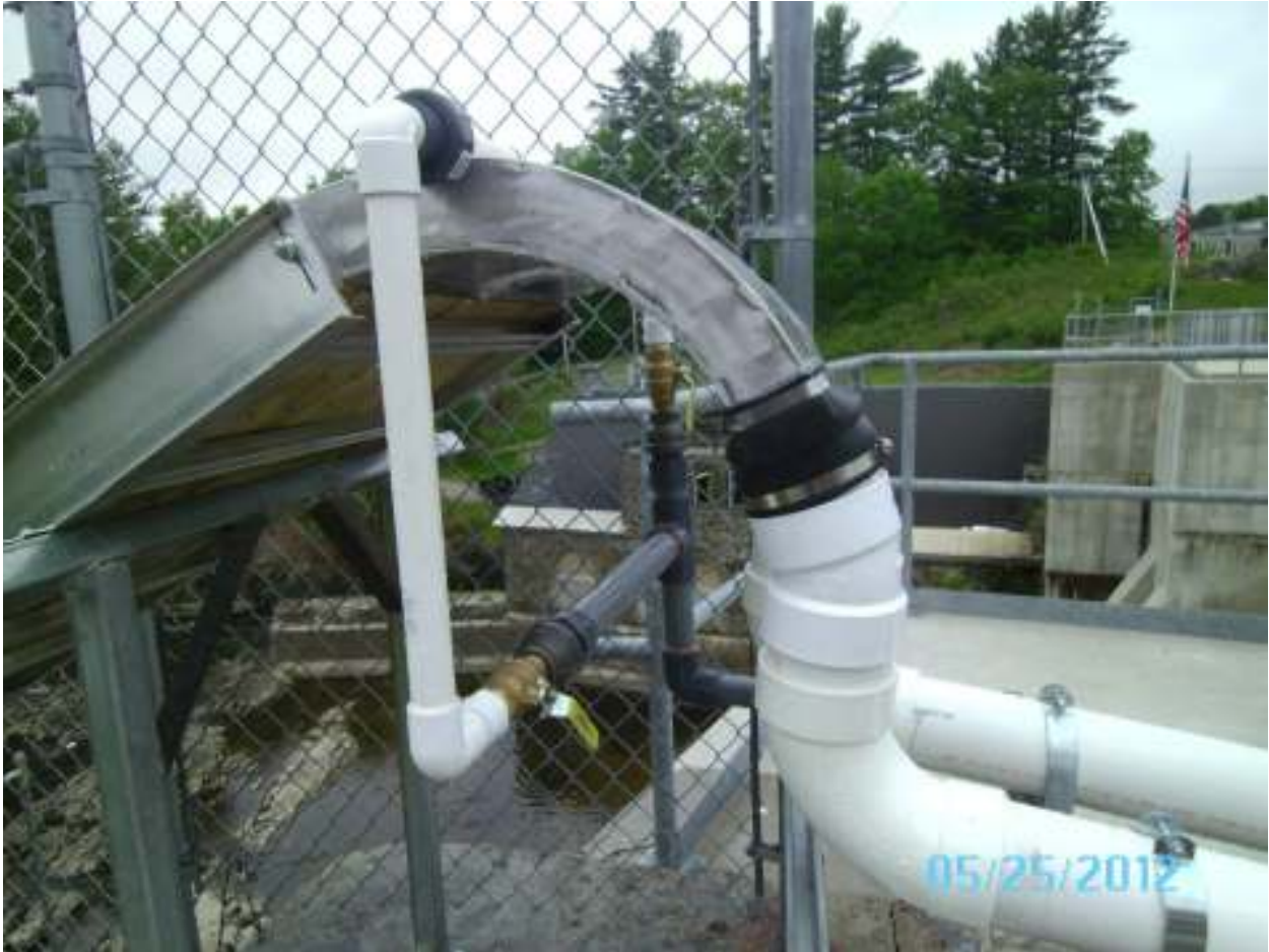
Terminal ends, spray bars, and head pond piping.
