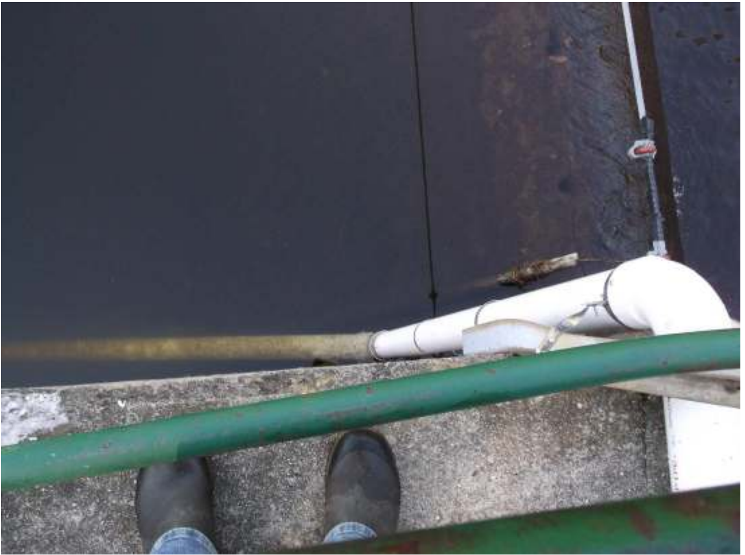
Fourteen ft. submerged exit pipe
