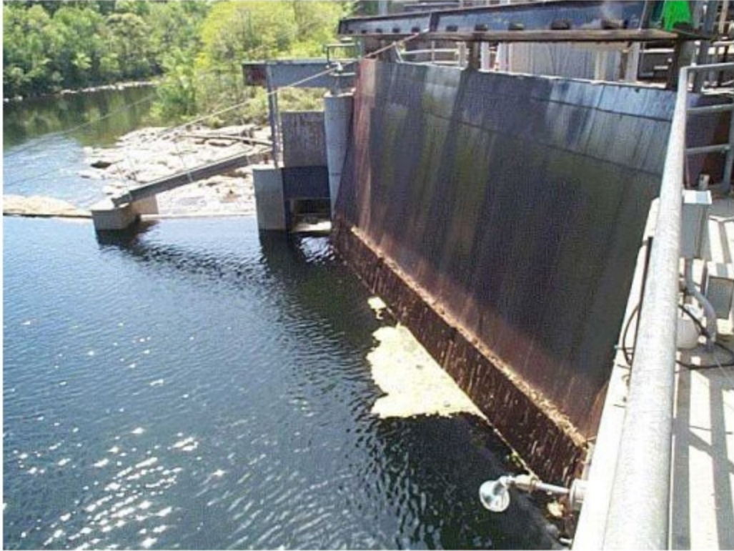
Figure 5 –Trashrack and Downstream Fish Passage Intake
