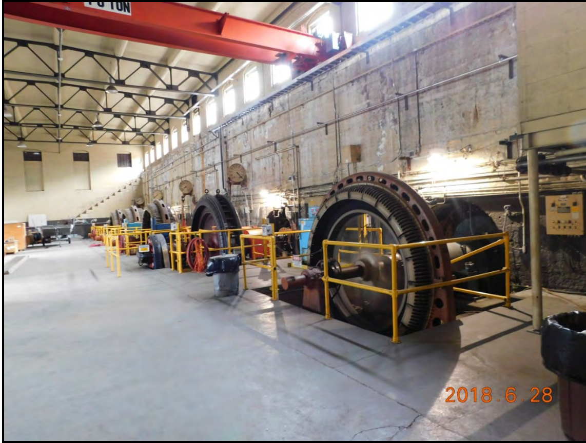
PHOTO 1-5 VIEW INSIDE THE CROSS POWER PROJECT POWERHOUSE.
