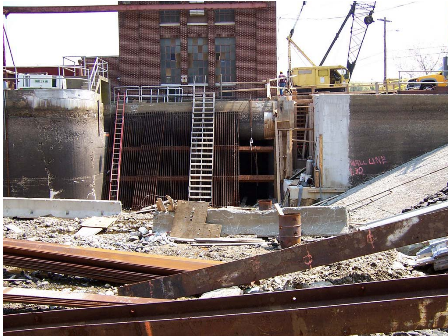
Photo No.5 - View of dewatered forebay area. Note downstream passage facility to right of trashracks.
