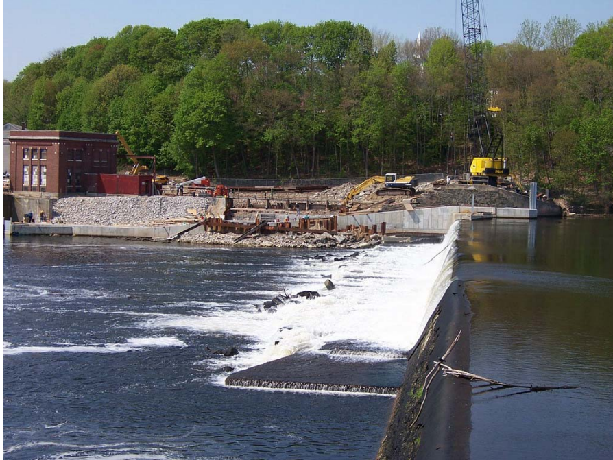
Photo No.1 - View of powerhouse and fish passage construction area from across the river.
