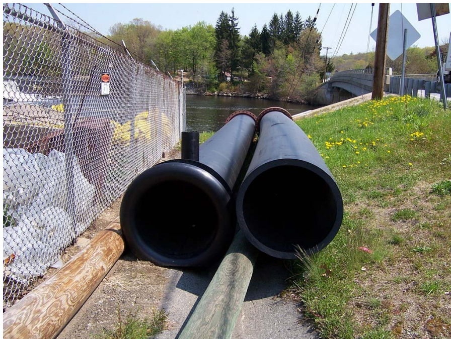
Photo No.6 - Discharge pipe for downstream fish passage, prior to installation.
