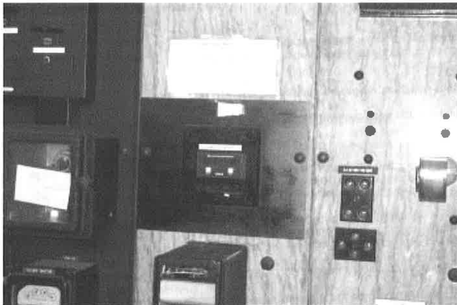
Photo No. 6 – View of the control panel in the powerhouse. The digital readout displays the headpond elevation which corresponds to the staff gage. (Not shown on Photo Location Map)
