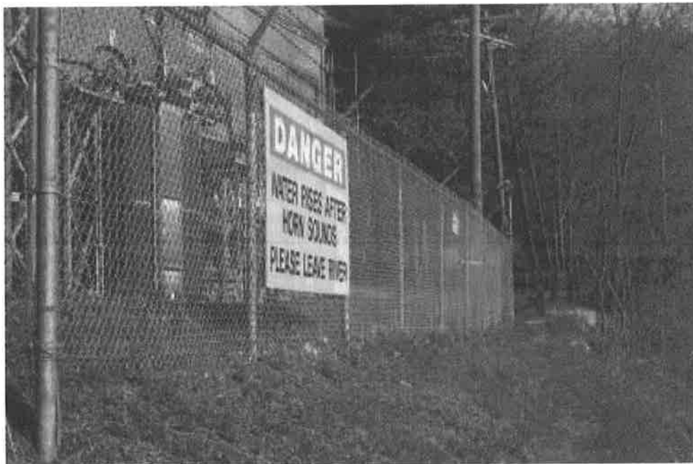
Photo No. 11 – View of the fence surrounding the powerhouse. Note “No Trespassing” sign posted along fence and more prominent sign warning of project flow releases.
