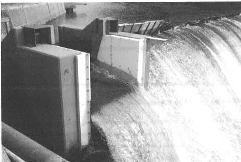
Photo No. 3 – View of the minimum flow release gate at the right side of the dam crest.
