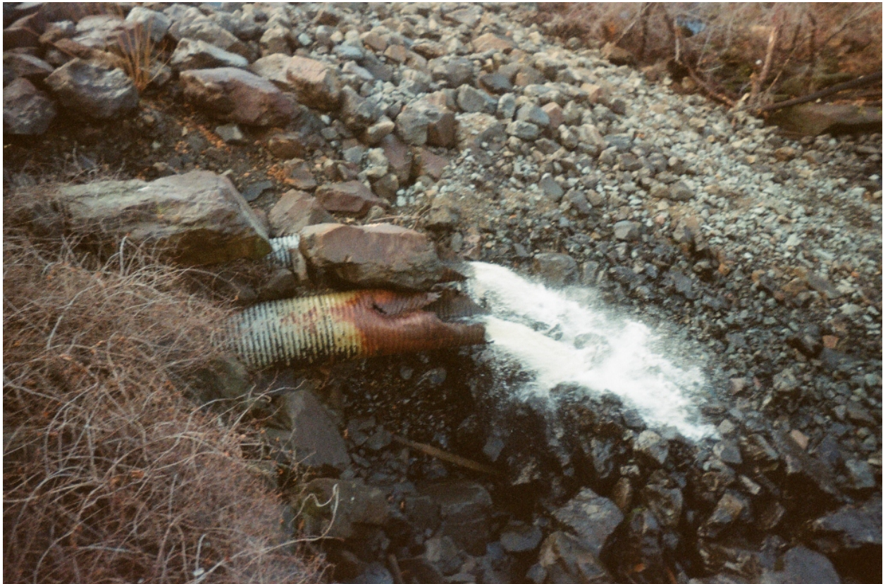
Minimum Flow Discharge Pipe (To Be Replaced by Year-end 2013)
