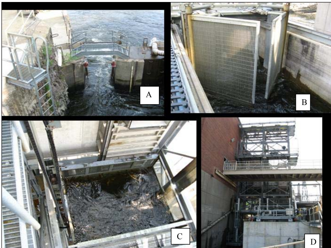
Figure 1-2. Holyoke fish lift, examples of components. A. tailrace east entrance (salmon gate), B. spillway fish lift crowder gate, C. Spillway fish lift hopper, full and raised nearly to exit flume elevation, D. fish lift towers viewed from downstream; the spillway lift is on the right.
