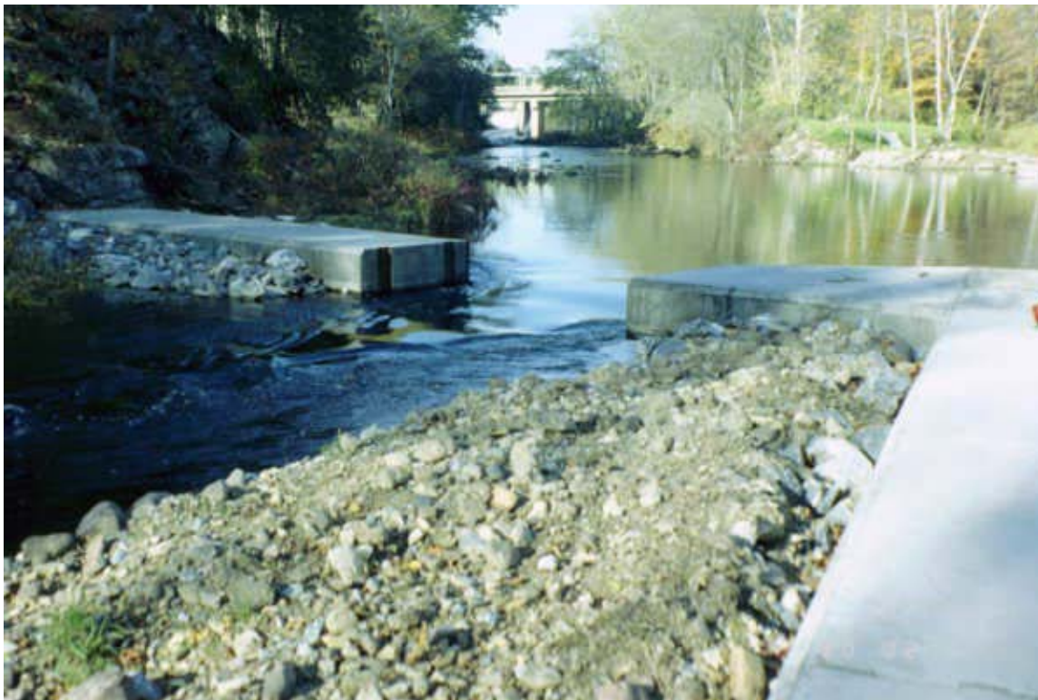
PHOTO 14 FLOW CONTROL WEIR (LOOKING UPSTREAM)
