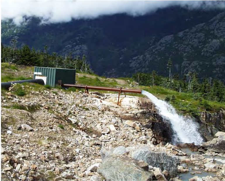
Figure 2. Valve house discharging aesthetics flow to Pitchfork Falls Creek.
