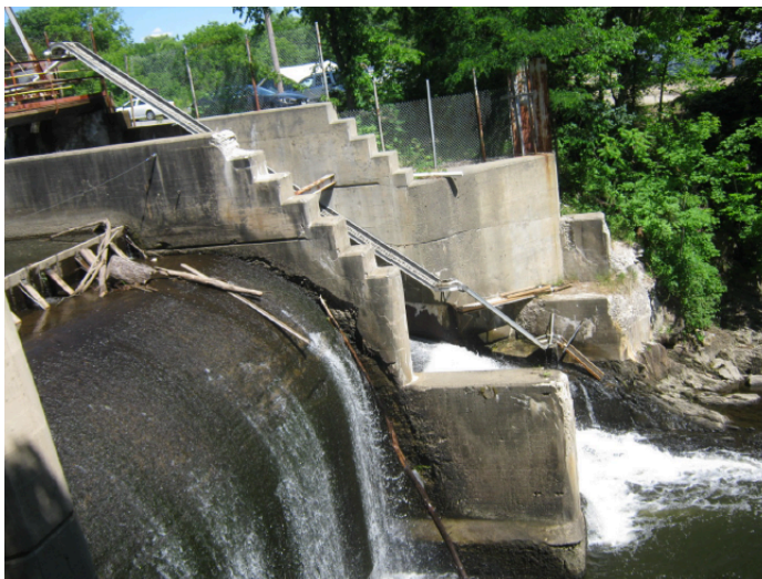
Figure 5. Eel ladder in place along left abutment.
