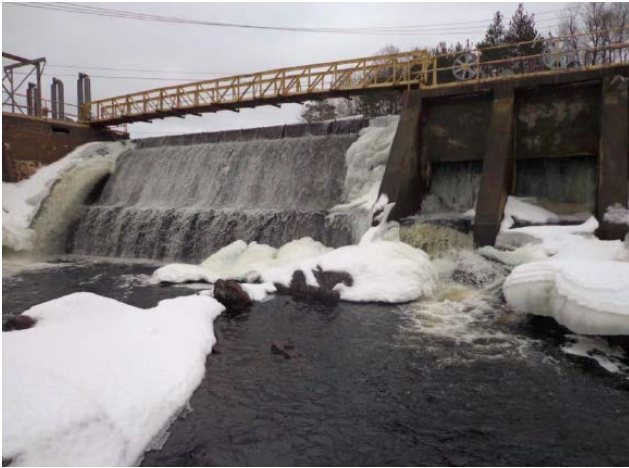
Figure 2 - Upper Newton Falls Minimum Flow Outlet
