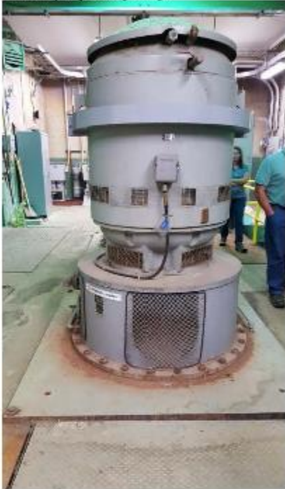
Figure 3: Secondary oil containment lip on pump motor approximately three quarters of the way up the pump.
