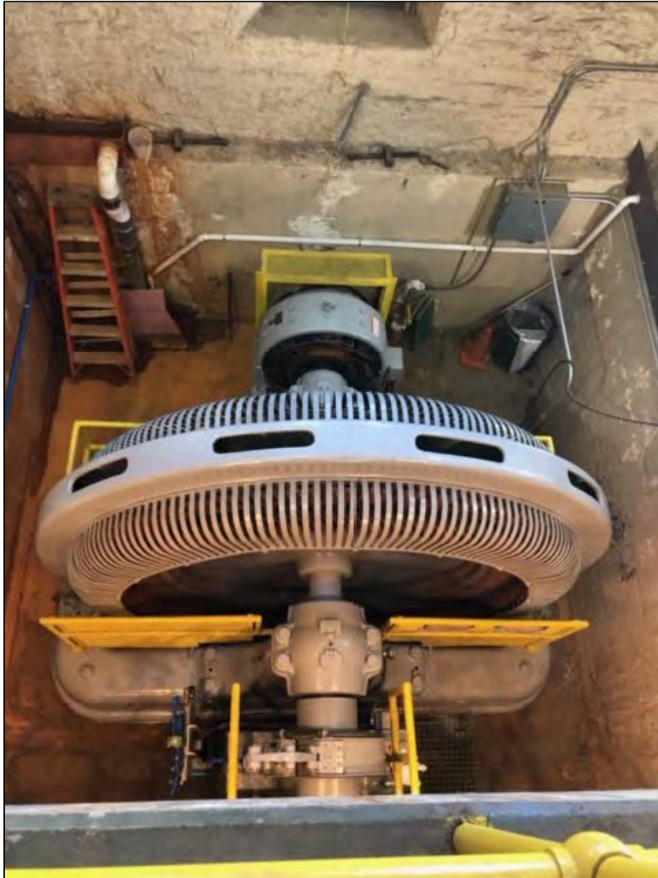
Figure 4 - View of Generator
