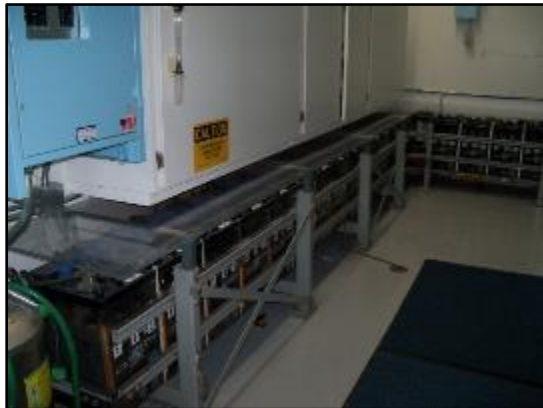
DC Battery Bank (left).
