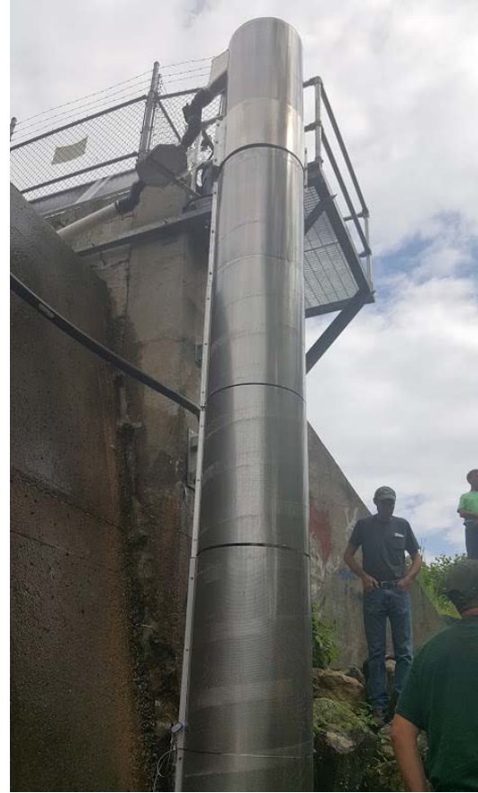
Eel ladder top section
