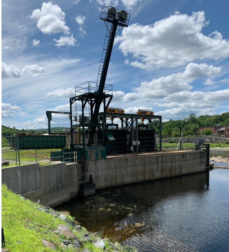
View of Powerhouse and Trash Rake (Looking Downstream)
