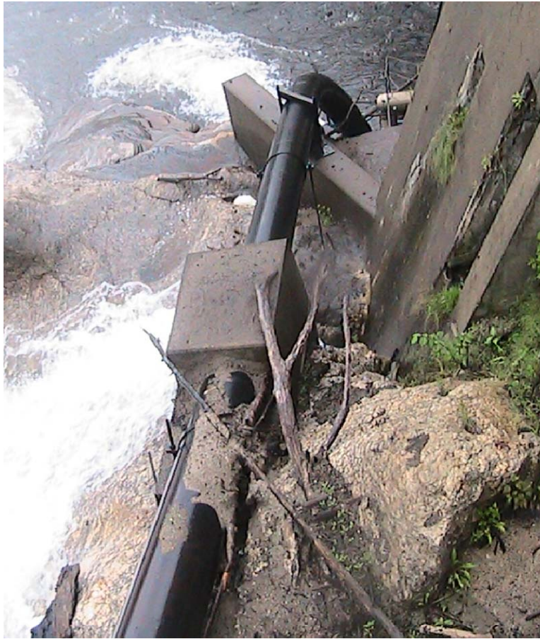
Photo 12G: Downstream Fish Bypass Pipe
