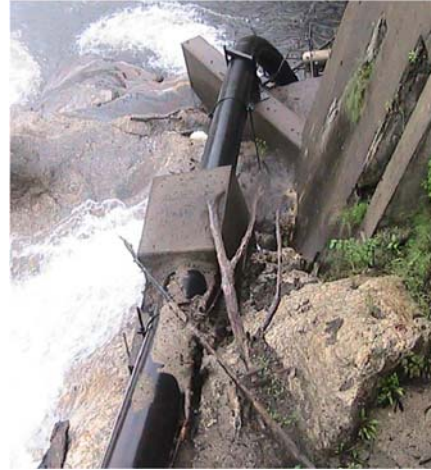
Figure 7 - Downstream Fish Bypass Pipe
