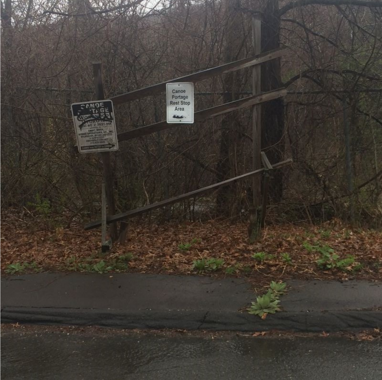
Portage rest stop in need of repair (photo taken on April 24, 2020)
