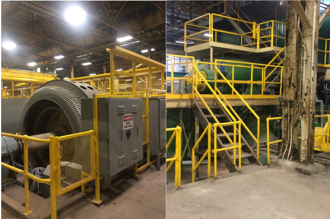
Millinocket Hydro Unit 6 Generator & Turbine
