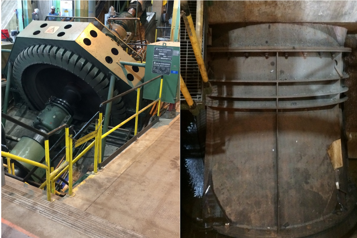
Dolby Unit 7 Generator & Turbine
