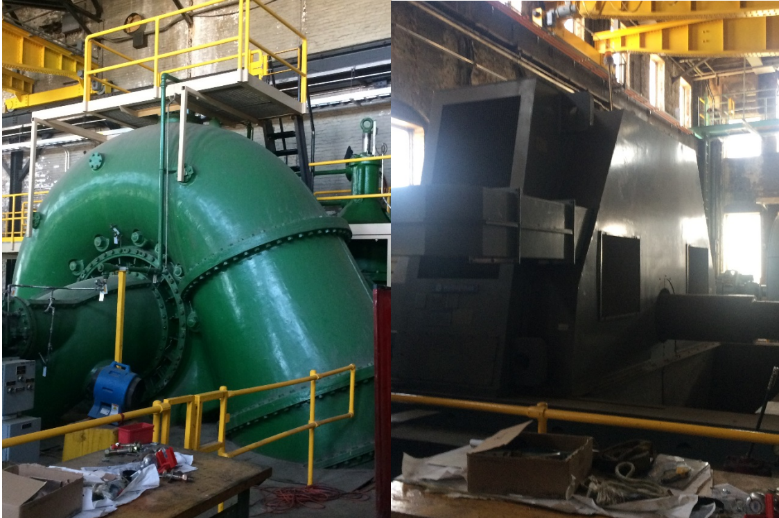
Millinocket Hydro Unit 8 Generator & Turbine
