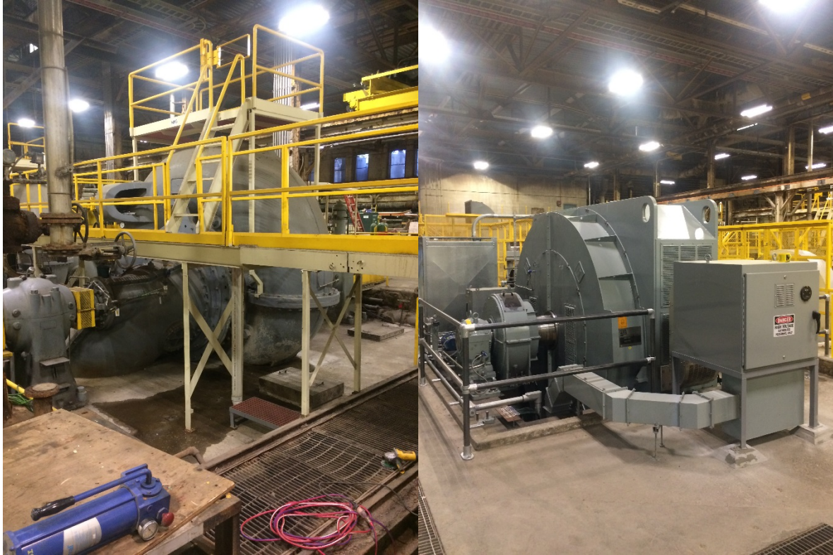
Millinocket Hydro Unit 3 Generator & Turbine
