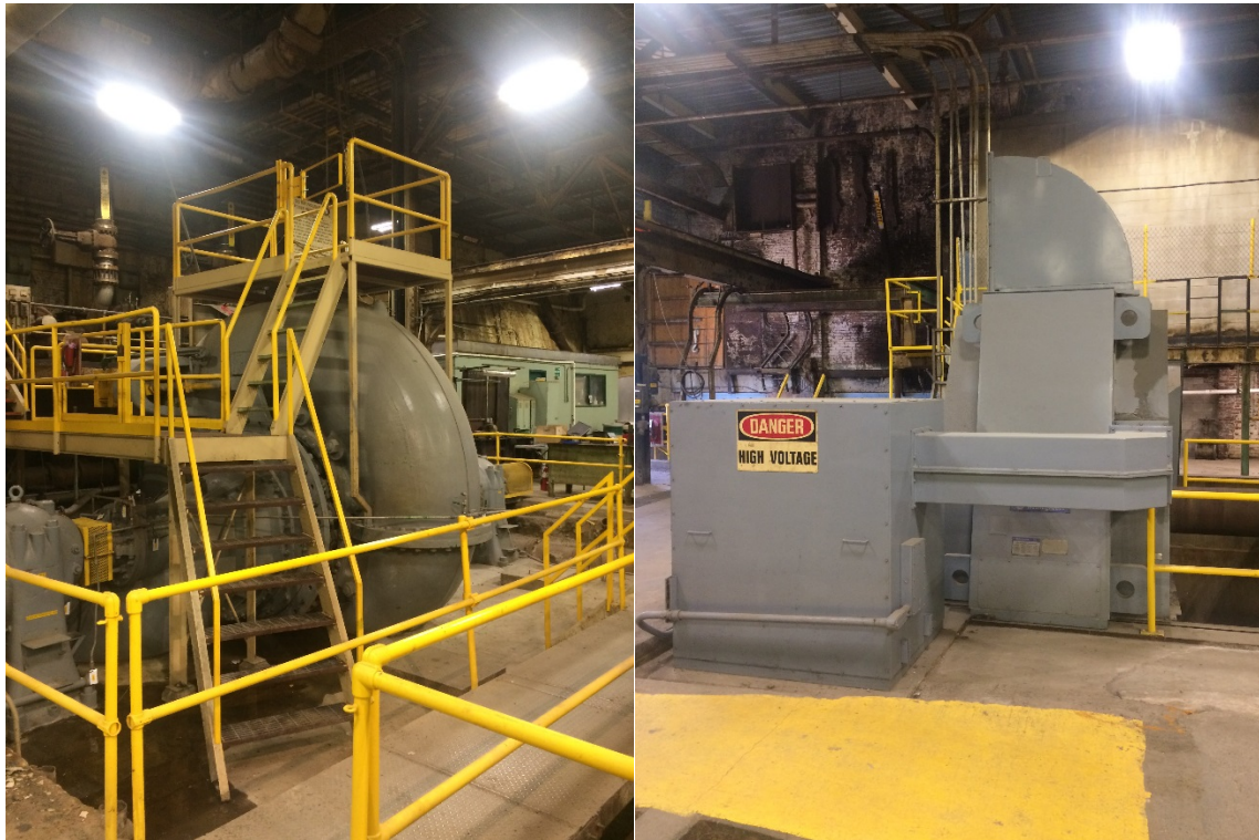
Millinocket Hydro Unit 1 Generator & Turbine
