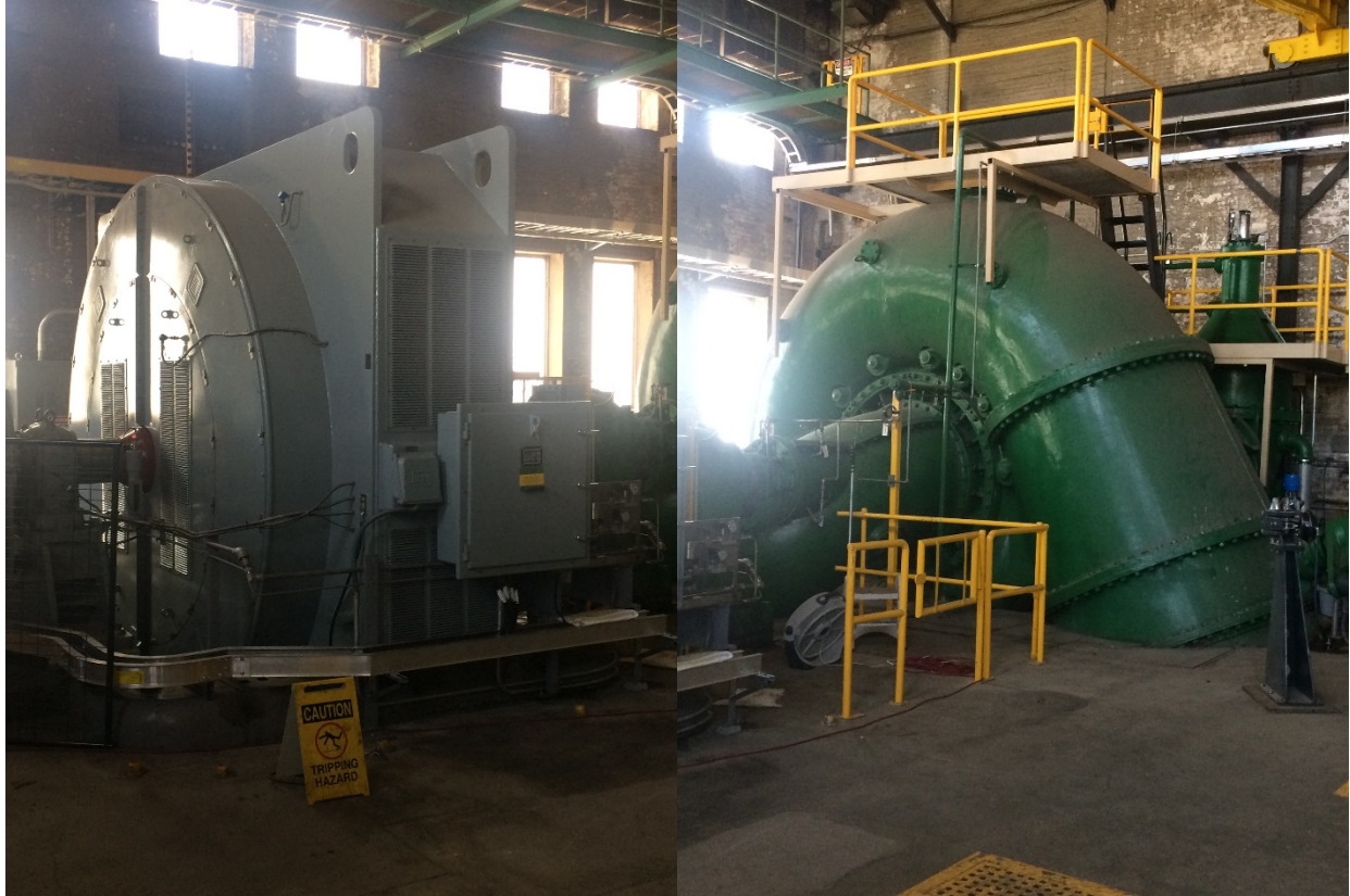
Millinocket Hydro Unit 7 Generator & Turbine
