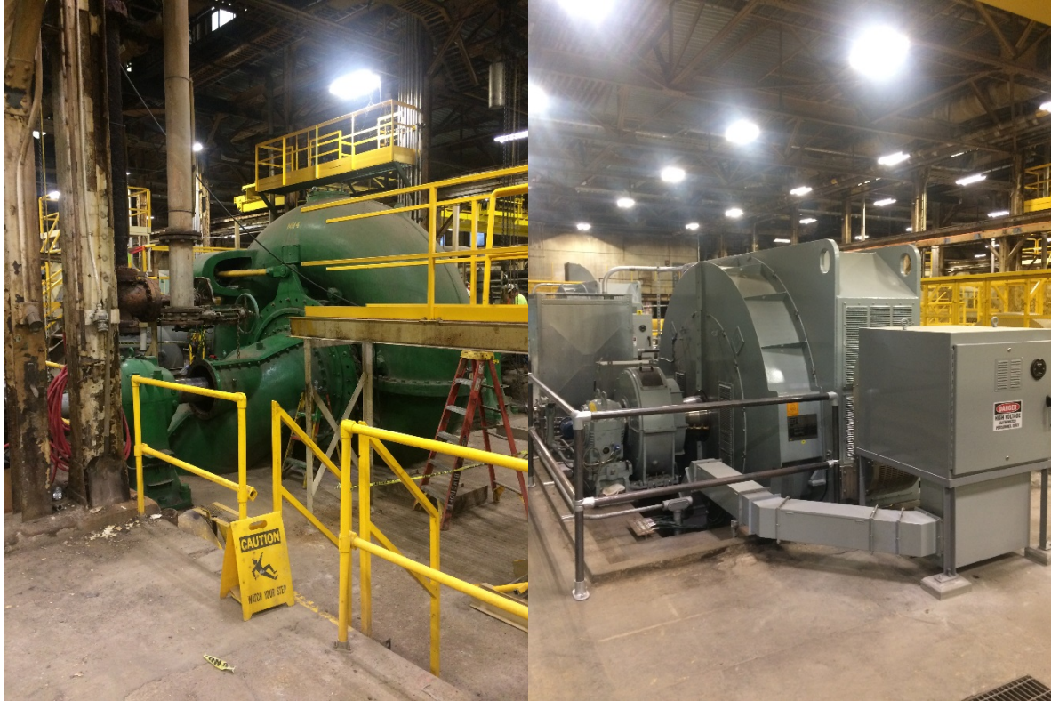
Millinocket Hydro Unit 4 Generator & Turbine
