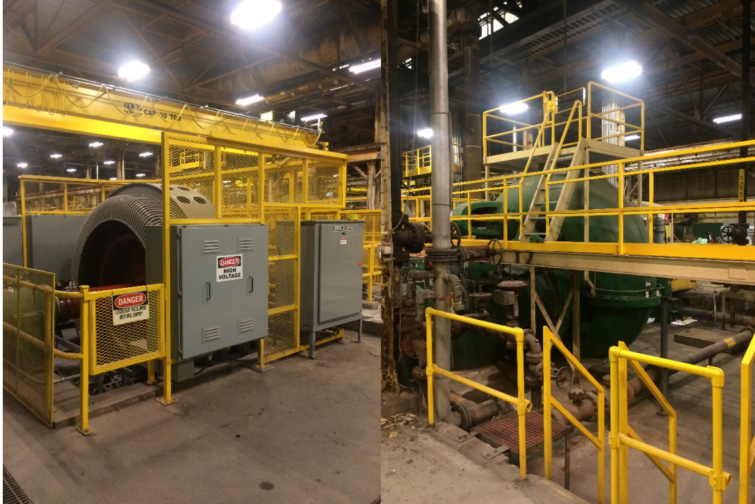
Millinocket Hydro Unit 5 Generator & Turbine
