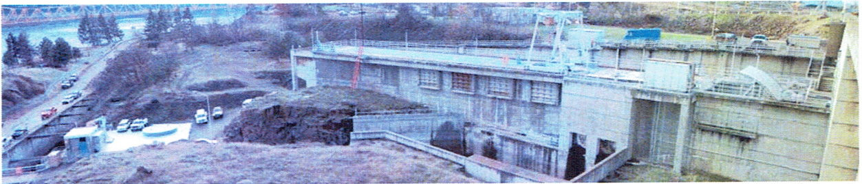
Photo 4. South side of the dewatering structure. The roof of the powerhouse is in the lower left corner of the picture.
