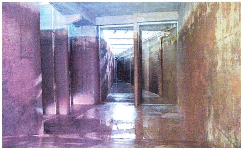
Photo 6. Interior view of the dewatering structure looking downstream. The diagonal wall screen is on the right.
