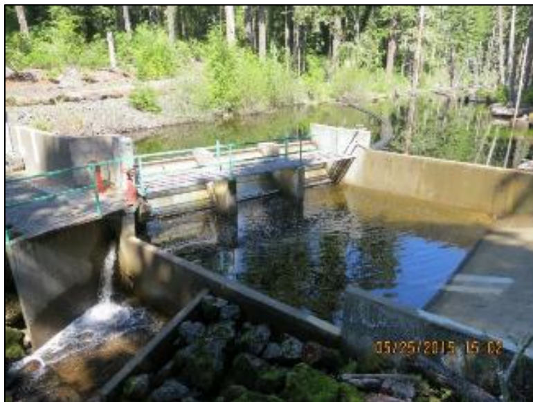
Figure 4: Diversion structure, showing weir and 1 cfs minimum flow discharge.
