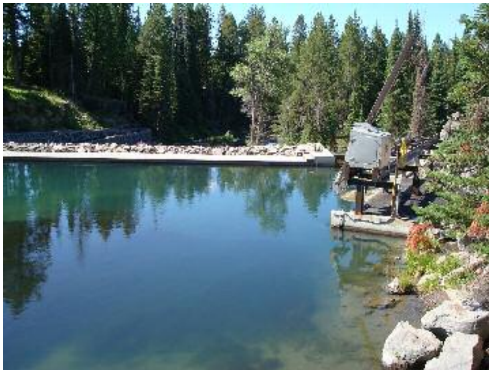
Photo 1: View looking south from the reservoir looking at the trashrack and automated rake on the right. The fishway is located in the background.
