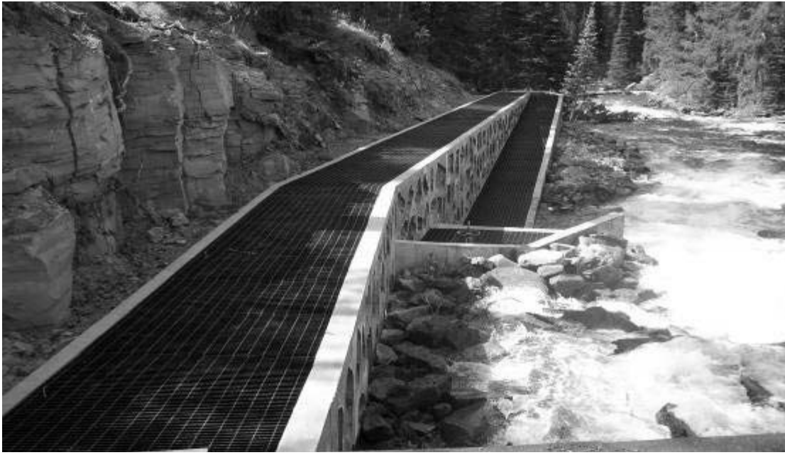
PHOTO 5 DOWNSTREAM VIEW OF PROJECT FISH LADDER
